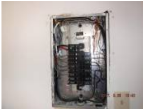
Subpanels- Detached Garage:
